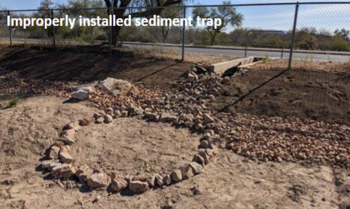
Improperly installed sediment trap
